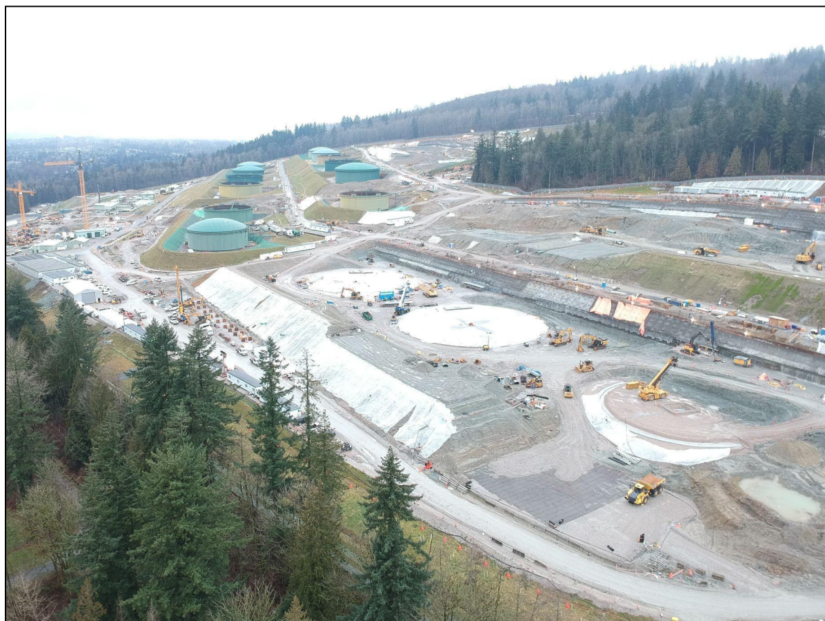
NOTE: Image 3) Photo of the Burnaby Terminal Expansion under construction. McCartney, Peter, 2021.
